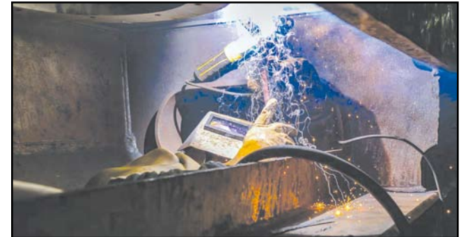
Newport News Shipbuilding contractor welds a bolt ring on the rim of a catapult cover on the flight deck of aircraft carrier John C. Stennis in Newport News, Va., in 2022. U.S. Navy photo by Jong S. Park
